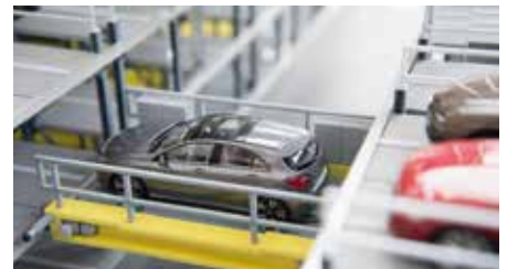
Opened in 2018 BLOX, COPENHAGEN, DENMARK Fully automated car park system with 350 parking spaces
